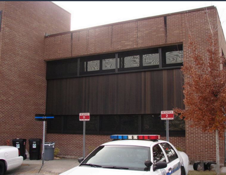
Fixed Screens protect upper levels of precinct.
