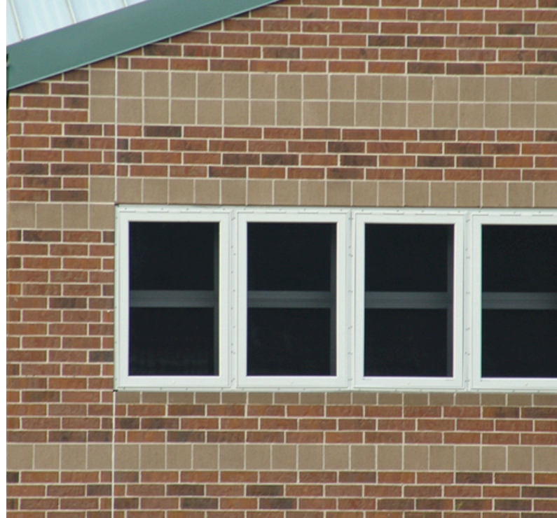
QMi security screens protecting windows at an elementary school.
