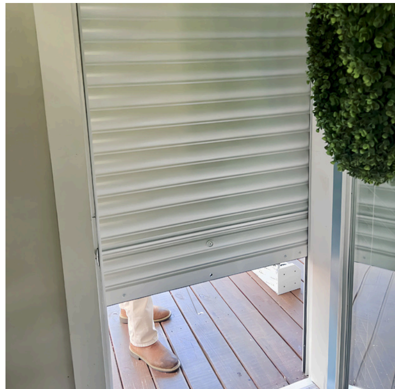
An exterior mounted Qcompact shutter being manually closed after being installed to protect the home's front door.
