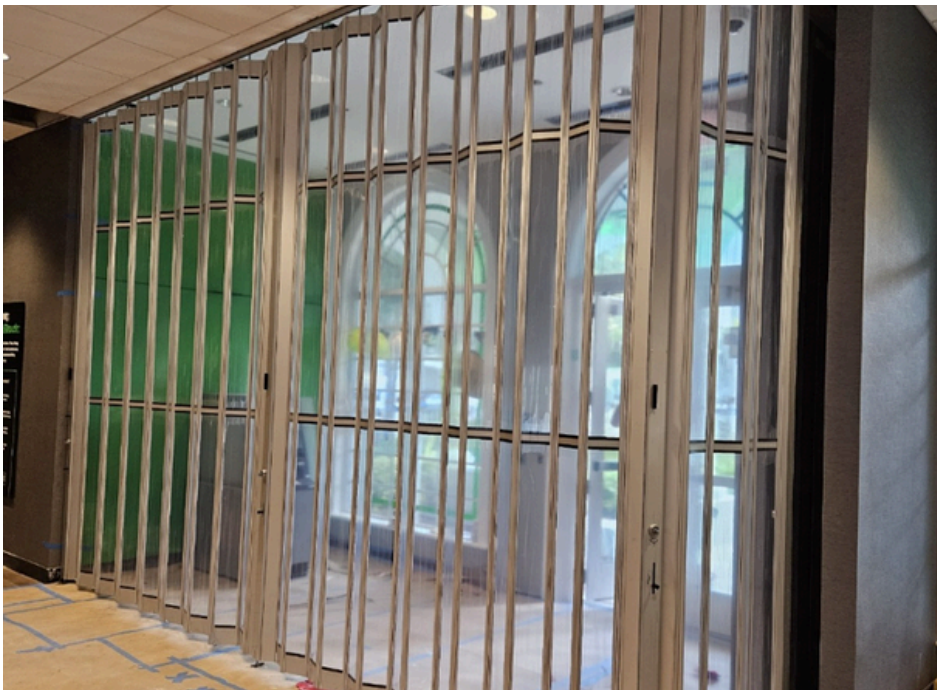
In-process installation of QMi Q-Clear Side-Folding Grille shipped with protective film over poly panels.
