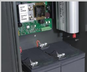
Two 35 Amp Hour SLA batteries fit inside the cabinet
